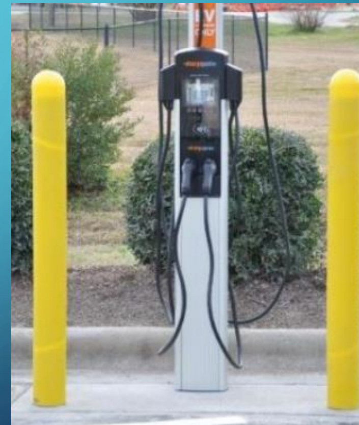
Level 2 Public Station
