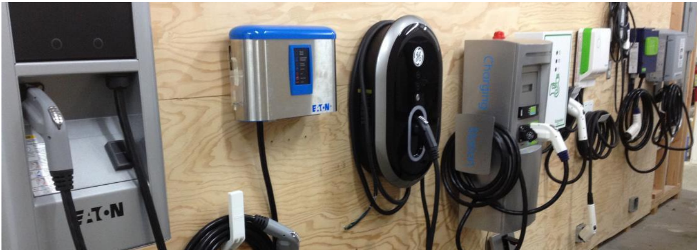
NW WA Electrical JATC EVSE Lab - Photo courtesy of Ryan Bradt
